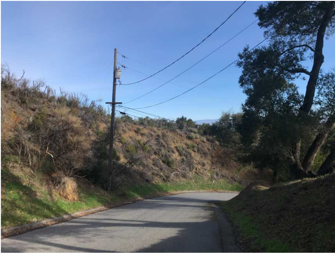
On private road looking at subject property (area of road cut mentioned in letter)
